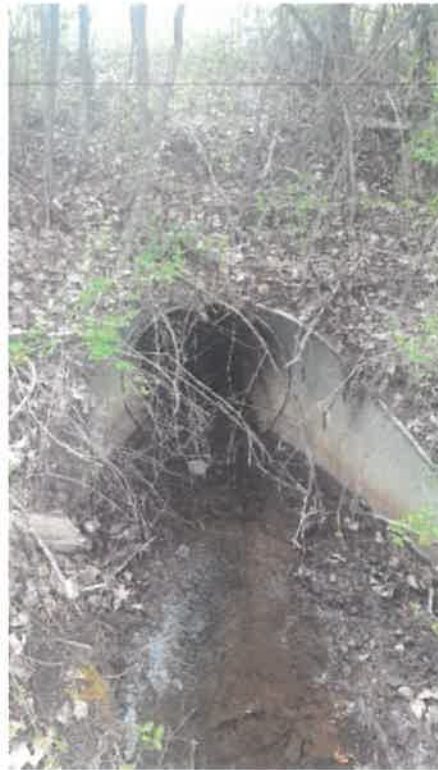
Photograph 8 – Culvert Inlet on Irrigation Canal on West Side of Creek at Highway 97
