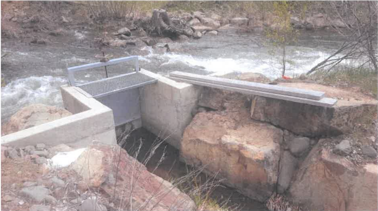
Photograph 1 - Diversion Structure with Slide Gate at Creek
