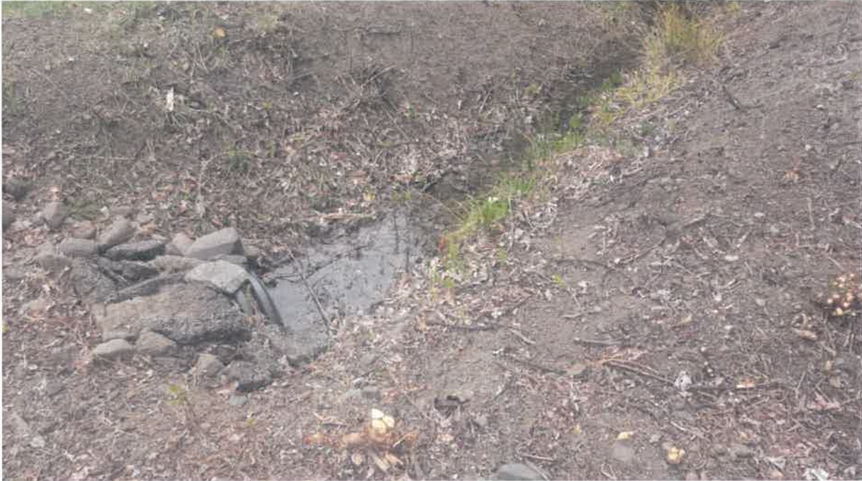
Photograph 9 – Upstream end of Culvert on West Side of Creek at Burke Road
